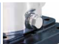
Measurements for suction and discharge pressure / drain
